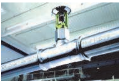
Stainless Steel pipework can be a quick & clean alternative to traditional materials
