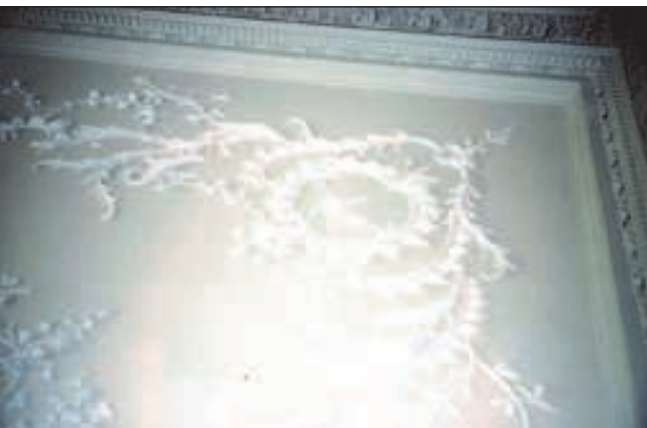
From the illustrations it will be seen that, with care and planning, sprinkler heads can be introduced into sensitive environments here aesthetic considerations are paramount.
