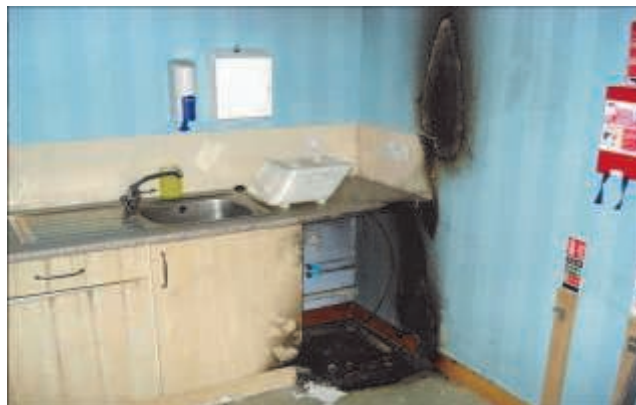
This picture shows the very limited fire damage after a single sprinkler head extinguished a fire. The fire was started by a dishwasher catching fire.
