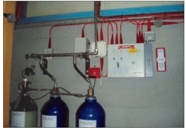
Water mist gas cylinders and manifold for a Hotel installation
