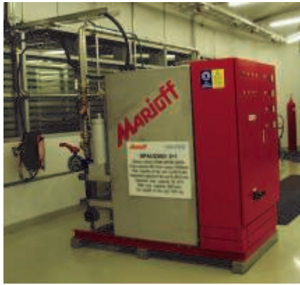
High pressure water mist pump set and control unit.
