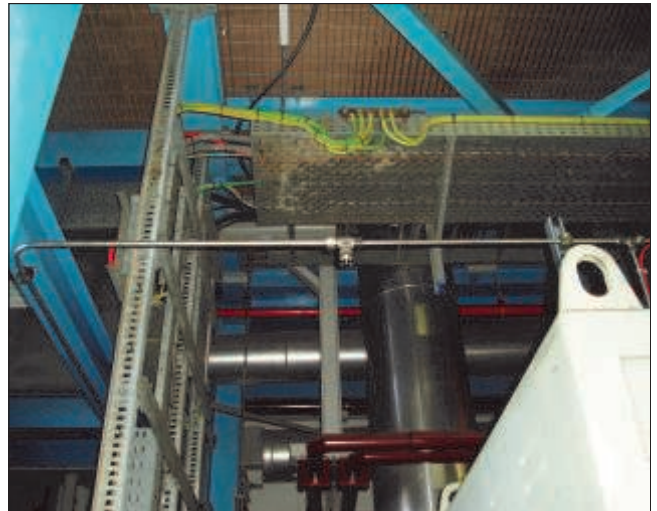
Mist nozzles and stainless steel pipework for a system in a power station
