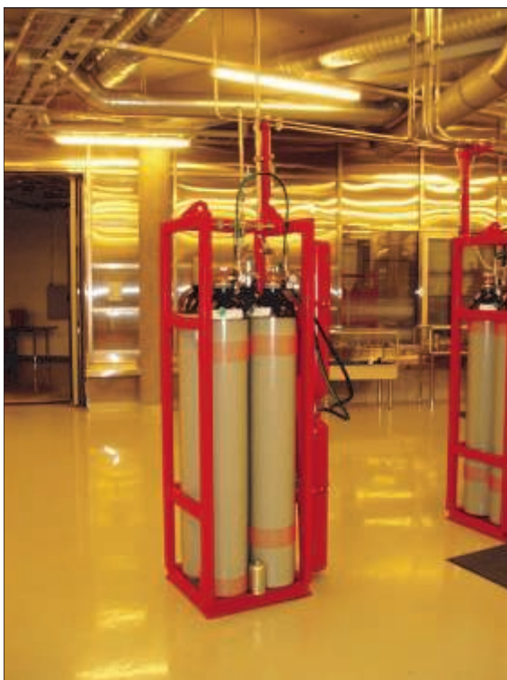
Replacement gas cylinders for a mist system
