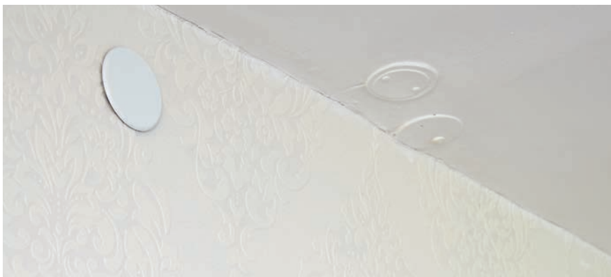
Cover plate fitted to sprinkler head
