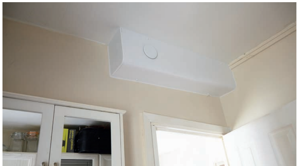
Preformed "Pendoc" boxing was used to cover the pipework inside the flats rather than locally constructed boxing used in other projects. This provided a far superior finish coupled with high quality caulking to stop gaps appearing following installation
