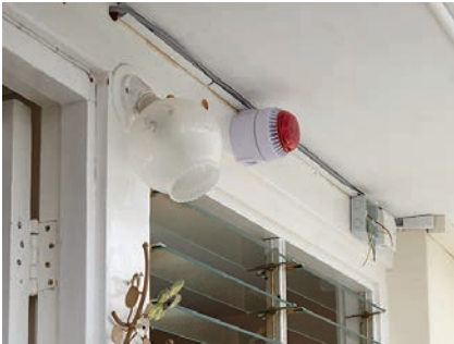
Electrical connections to alarm and sounder
