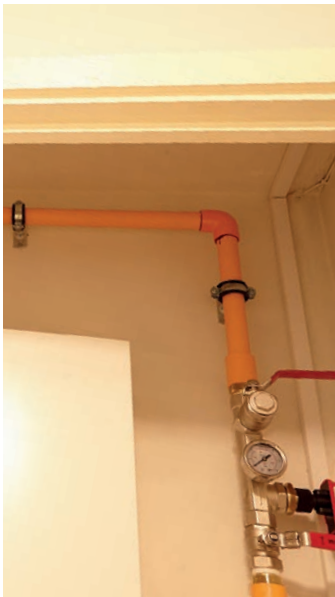
Isolation valve, gauge and flow switch in individual property
