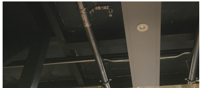
Interior showing complex ceiling decor with mist nozzle. Pipework is visible to avoid fabric damage.
