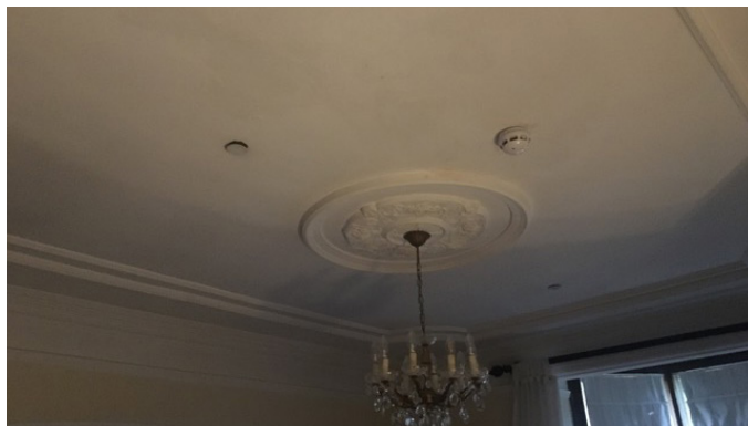
Two pendant concealed heads protect this large bedroom
