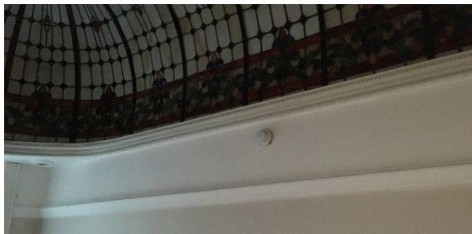
Sidewall sprinkler head protecting a 4m x 4m hotel bedroom.
