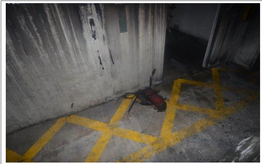
Figure 3.4.8 Remnants of Fire point, Level 3 Stairwell 3
