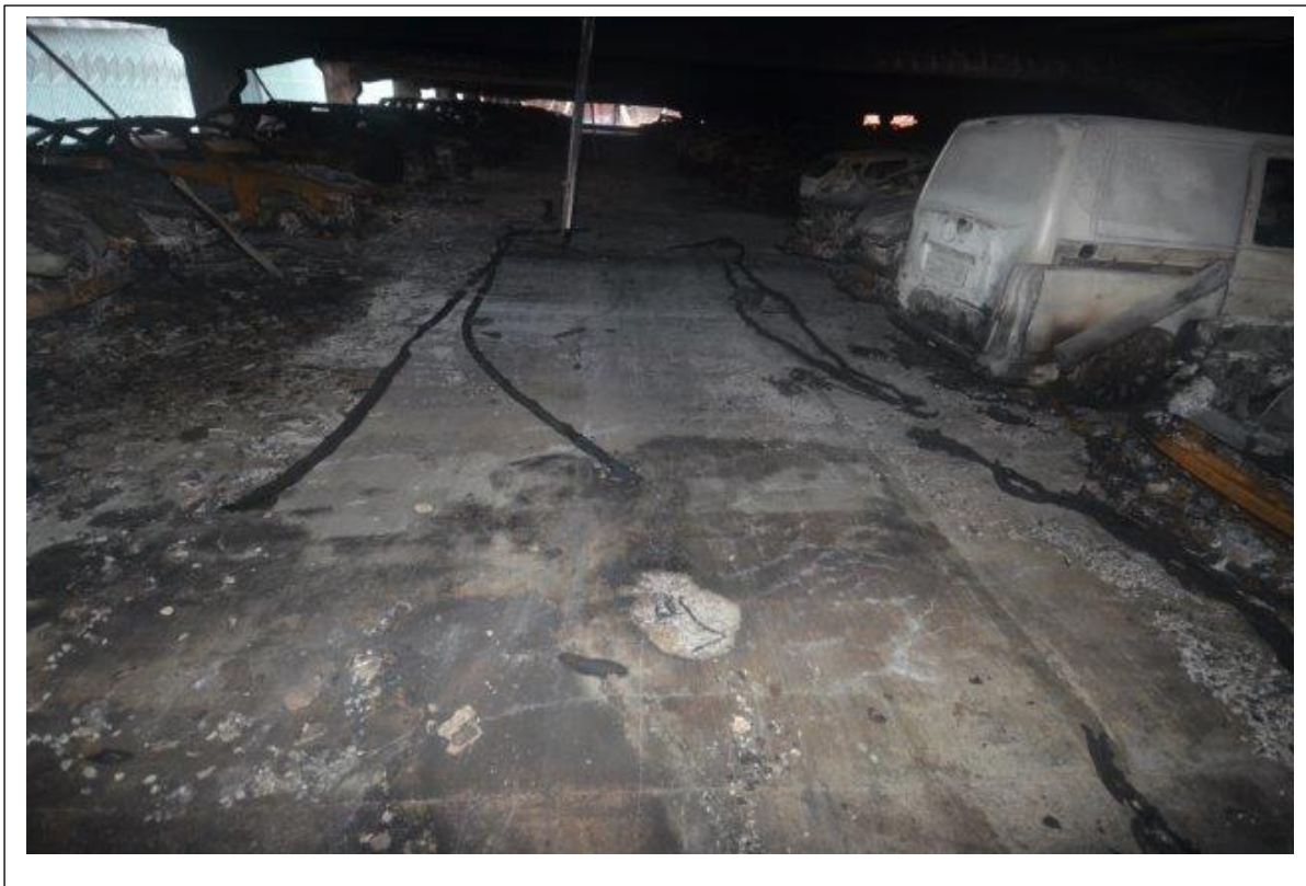
Figure 2.4.1: Photograph of Spalled Concrete: Level 3
