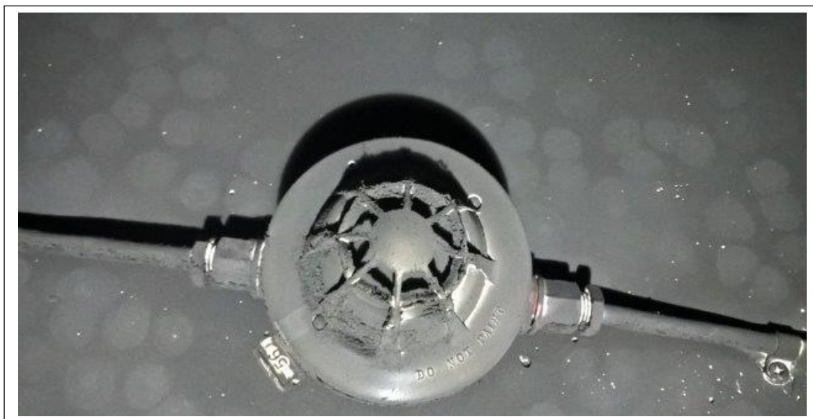
Figure 3.4.5: Photograph of Multi-sensor in Lift Lobby, Stairwell 2, Level 3
