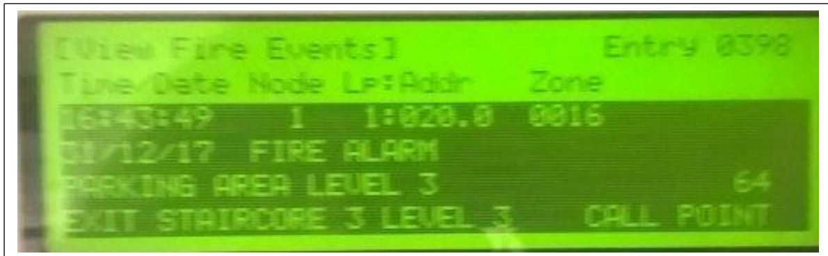
Figure 3.4.2: Photograph of Alarm Panel, 1st Actuation
