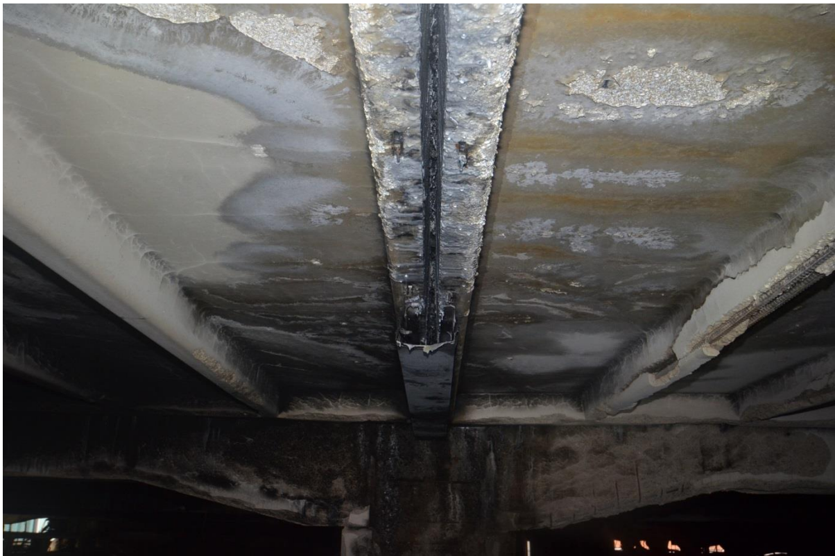
Figure 2.2.6: melted aluminium drainage tray and visible drainage slot
