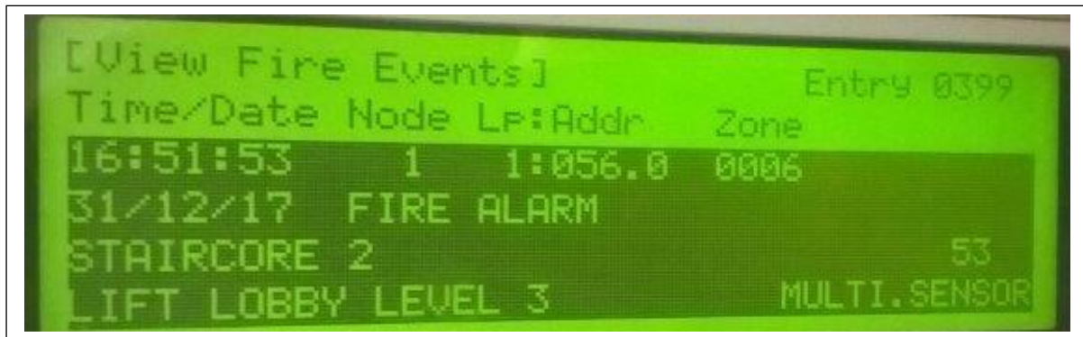
Figure 3.4.4: Photograph of Alarm Panel, 1st Actuation
