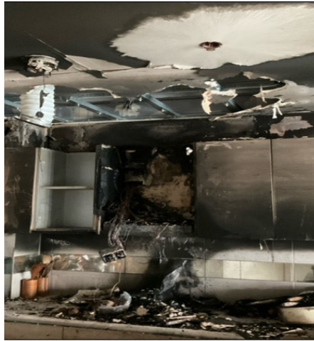
Kitchen extractor fan/wall units damaged by fire Credit tptfire
