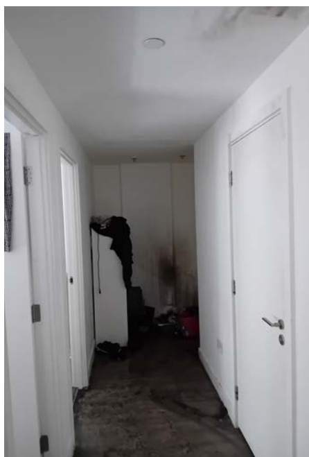
Internal hallway of flat identifying the location of the fire. Credit AFRS
