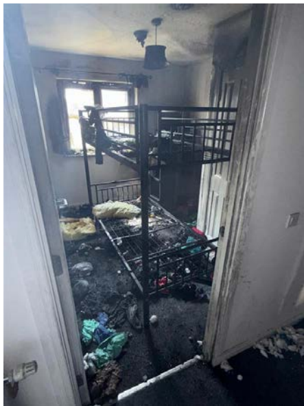
Internal view of the fire within the children's bedroom extinguished by the water mist system. Credit Imist™
