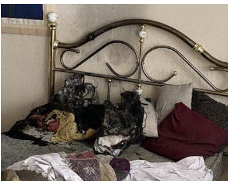
Bed damaged by fire. Credit BM Sprinklers/Triangle
