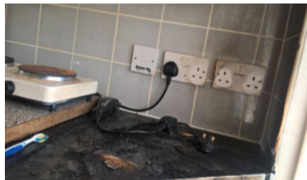
View of toaster identifying the seat of the fire. Credit Image LFB
