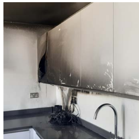
Seat of the fire identifying the burnt-out electric air fryer located on the kitchen work top and distinctive smoke layer. Credit AFRS
