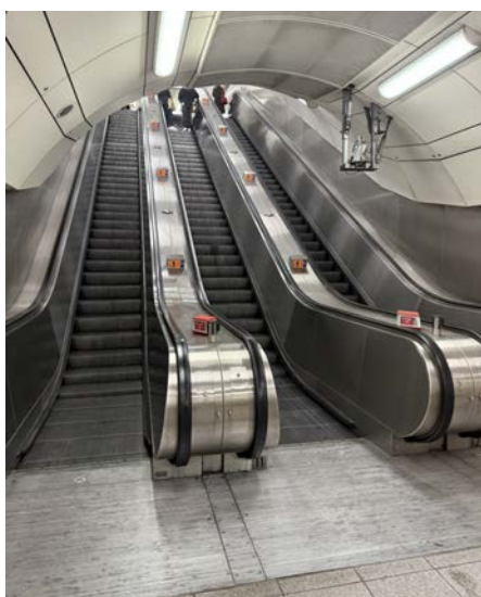
View of a typical London underground metal escalator
