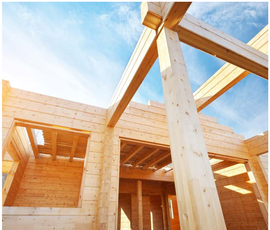
In Finland, buildings can use wooden construction at 4-8 storeys only if protected with sprinkler
