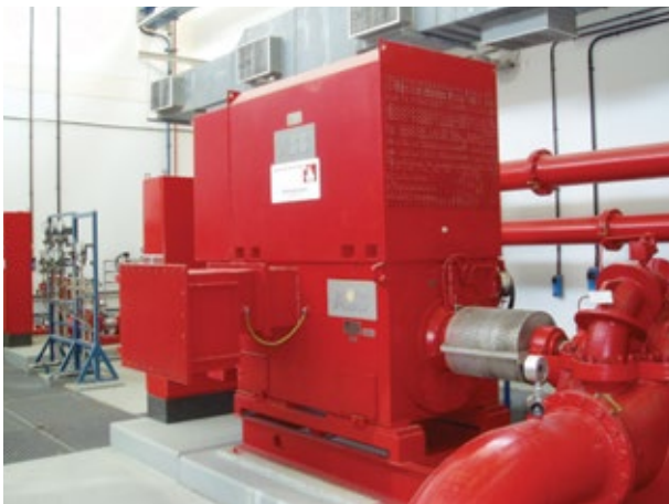
Large electrically-driven pump with coupling protection
