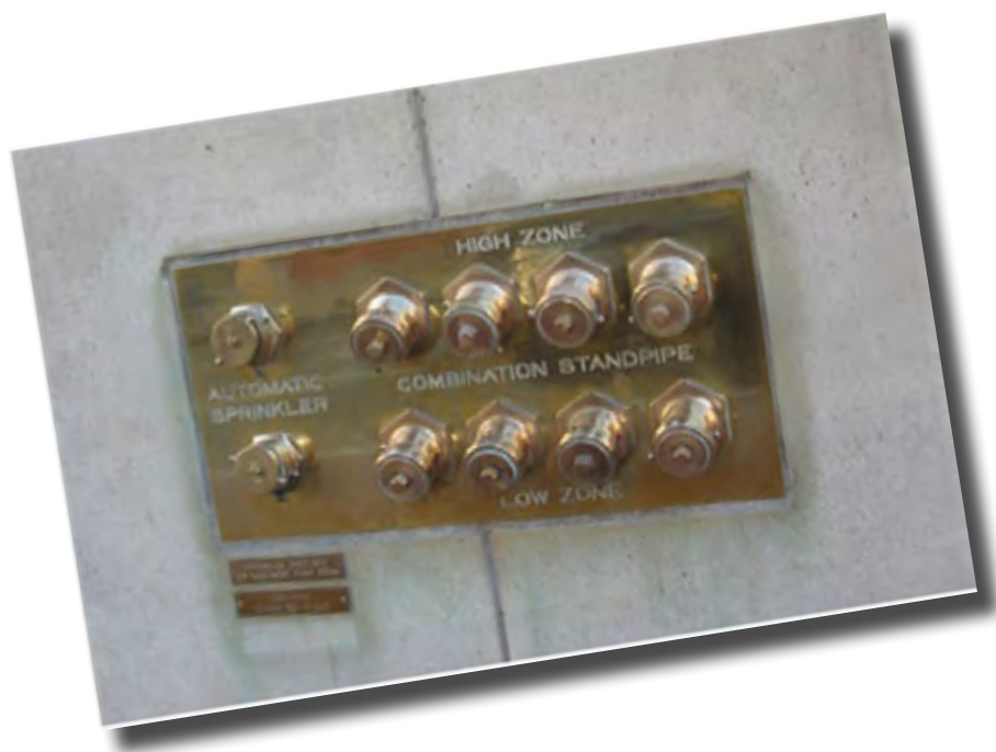
Streetside sprinkler evidence. This shiny fire service inlet was snapped on a high-rise building near Union Square, San Francisco.
