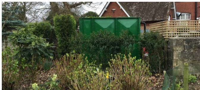
Modular GRP sprinkler water tank in listed hotel
