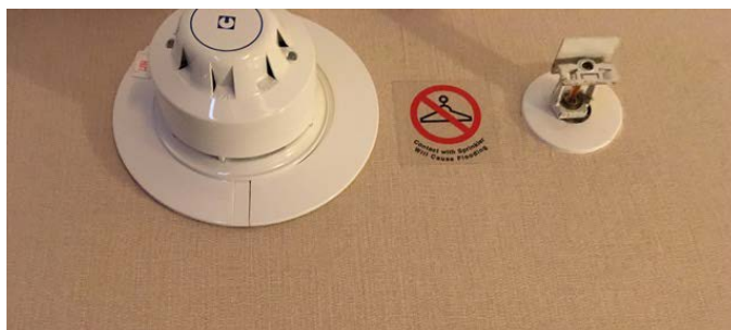
Retrofitted sprinkler system in an Grade II* hotel in Bristol. Note that warning sign - garment bags and sprinklers are not friends!
